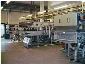
Professional, preventive inspection and maintenance, also process optimisation for minimisation of operating costs
