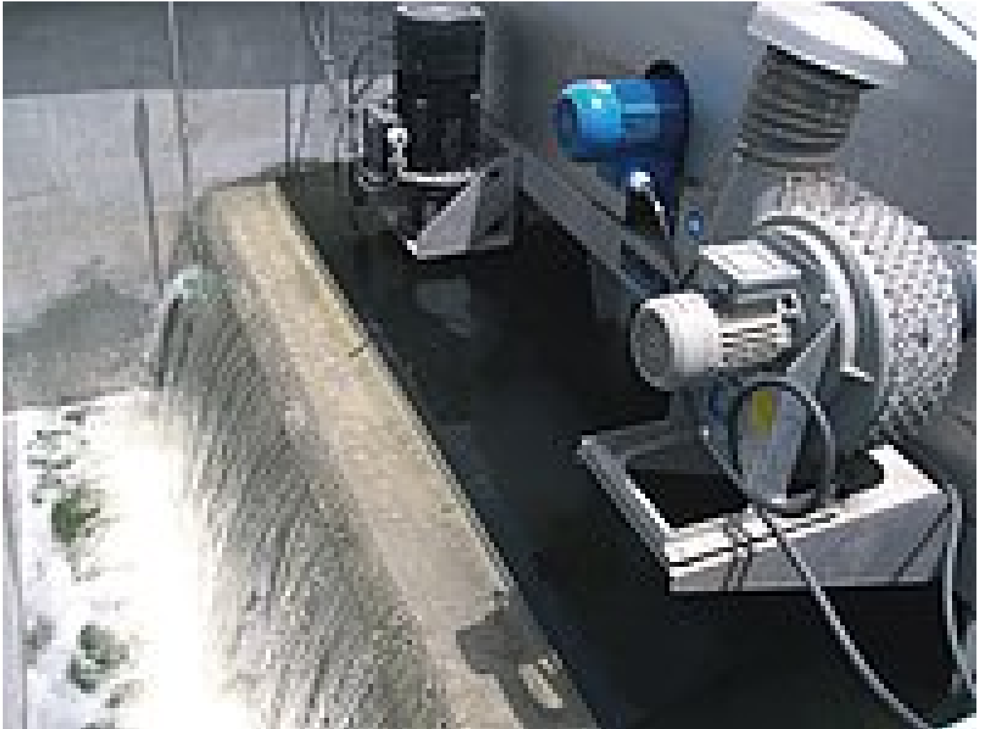
Effluent from our RoDisc® 20 micro-screens
