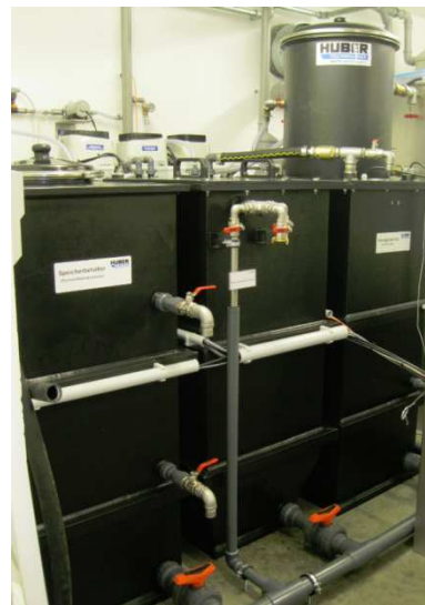
HUBER MBR greywater treatment plant
