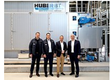
A showcase project that stands for the highest art of engineering: commissioning the HUBER Belt Dryer BT 16 at WWTP Erlangen
